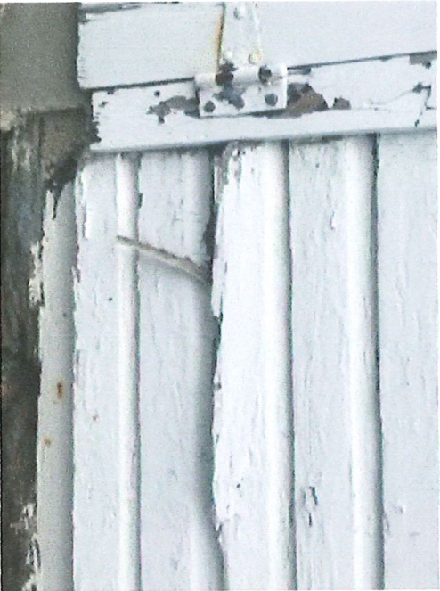
Original rotting German siding at bottom and up the walls. This includes damage from rain and other moisture.
